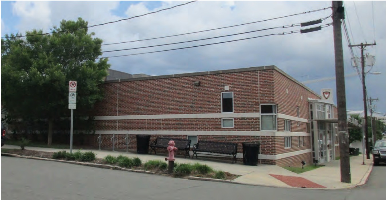
Figure 75: Rigsbee Avenue Substation
