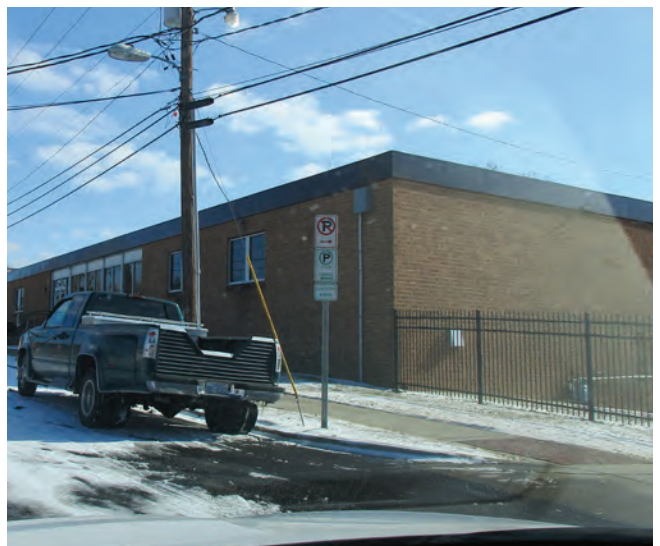
Figure 64: Rigsbee Avenue Substation
