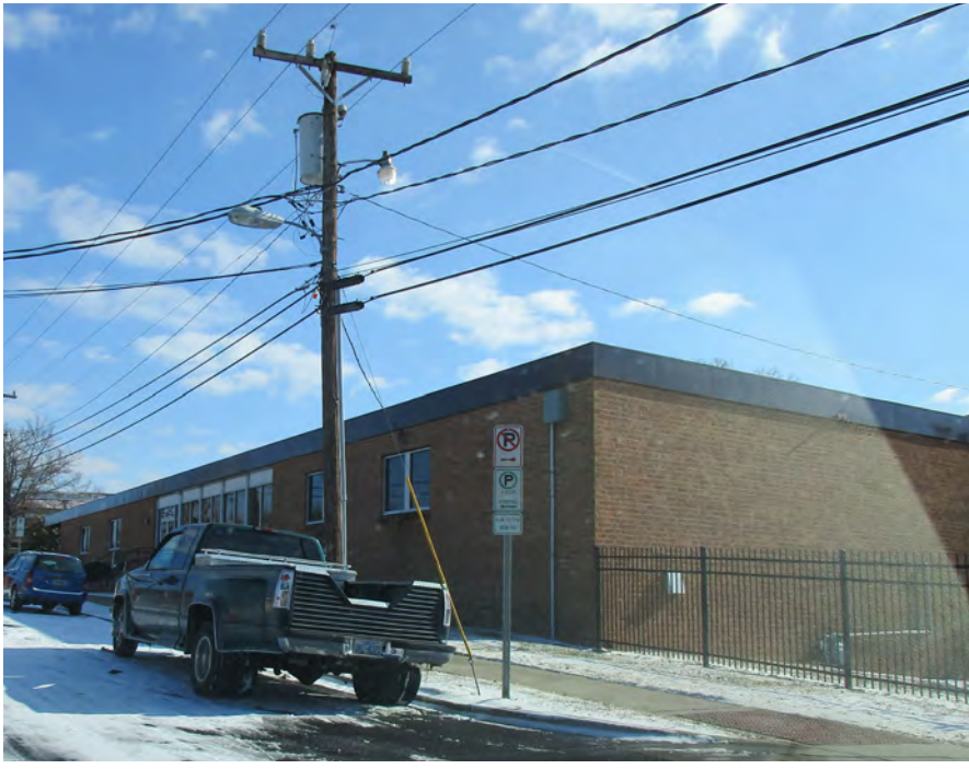
VIEW OF RIGSBEE AVENUE SUB-STATION
